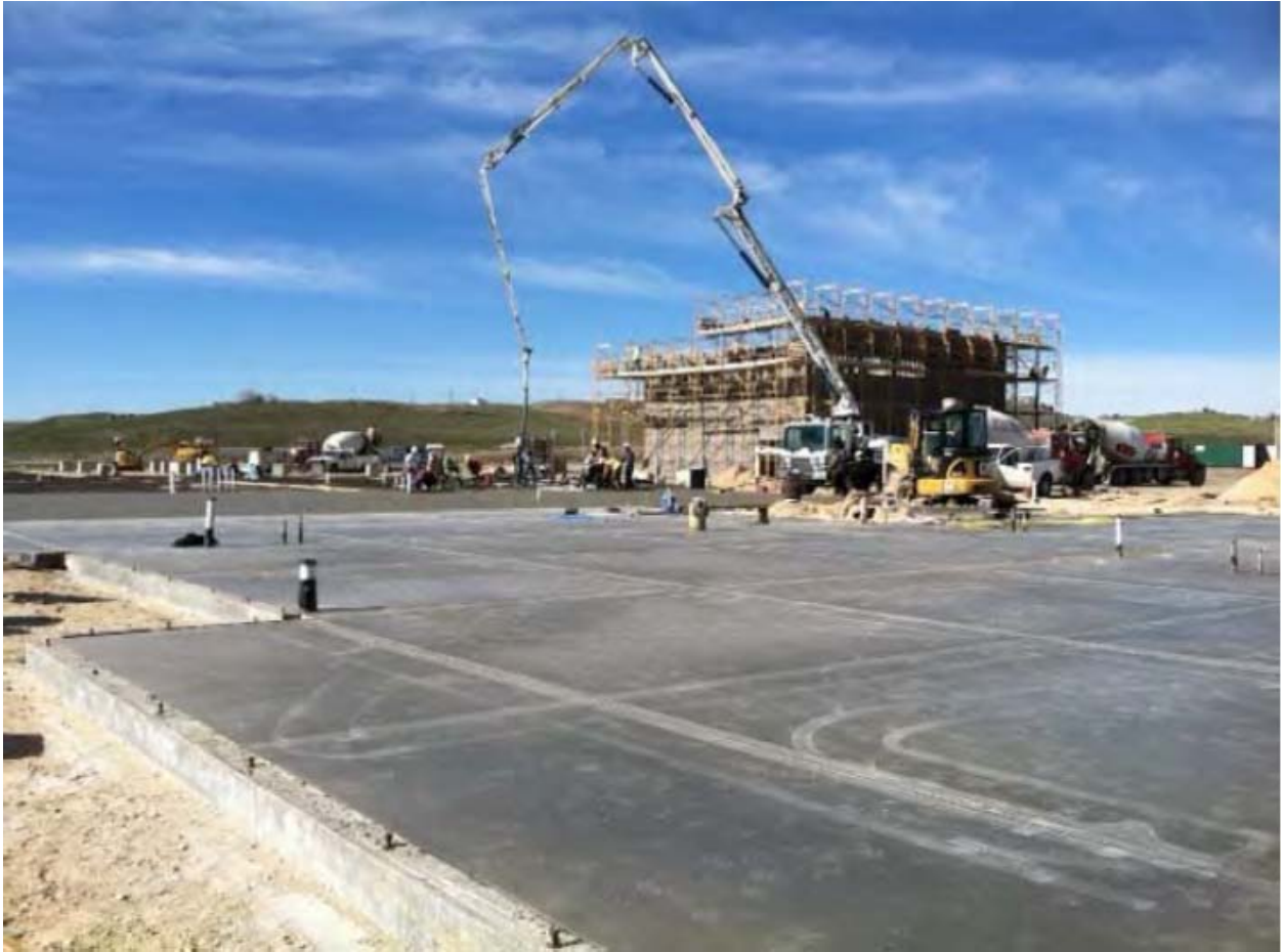
April 2014- Overall site – Pumping concrete for slab with Workforce Training Lab in background
